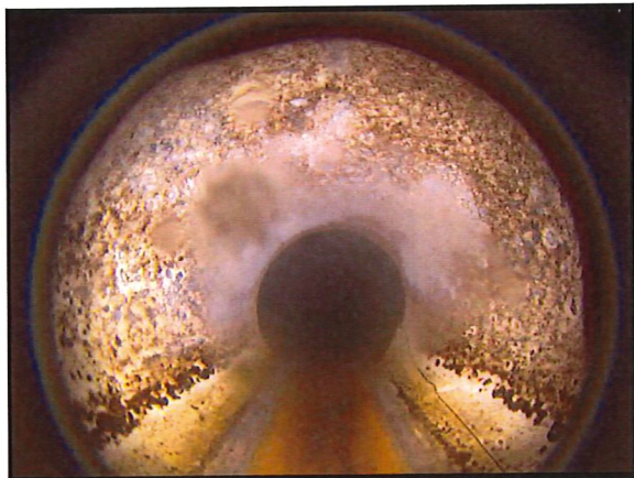
Figure 19: PS10_P065; Condition: 3; Spiral Crack
