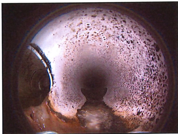
Figure 7: GP2_P019; Condition: 4; Deposits: Water Jet
